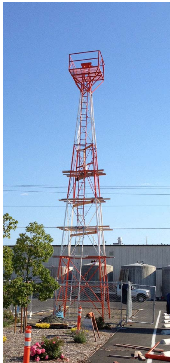
The tower has a top thanks to Ron Price. Next up, the airway beacon to go on top.
